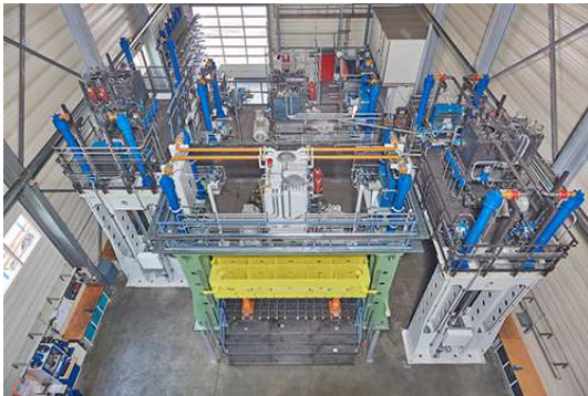
Image 1: Intelligent press from Schnupp achieves power and precision by means of four Rexroth hydraulic axes. Four machines have been set up for pre-assembly in a very confined space. (Copyright: Bosch Rexroth AG)
